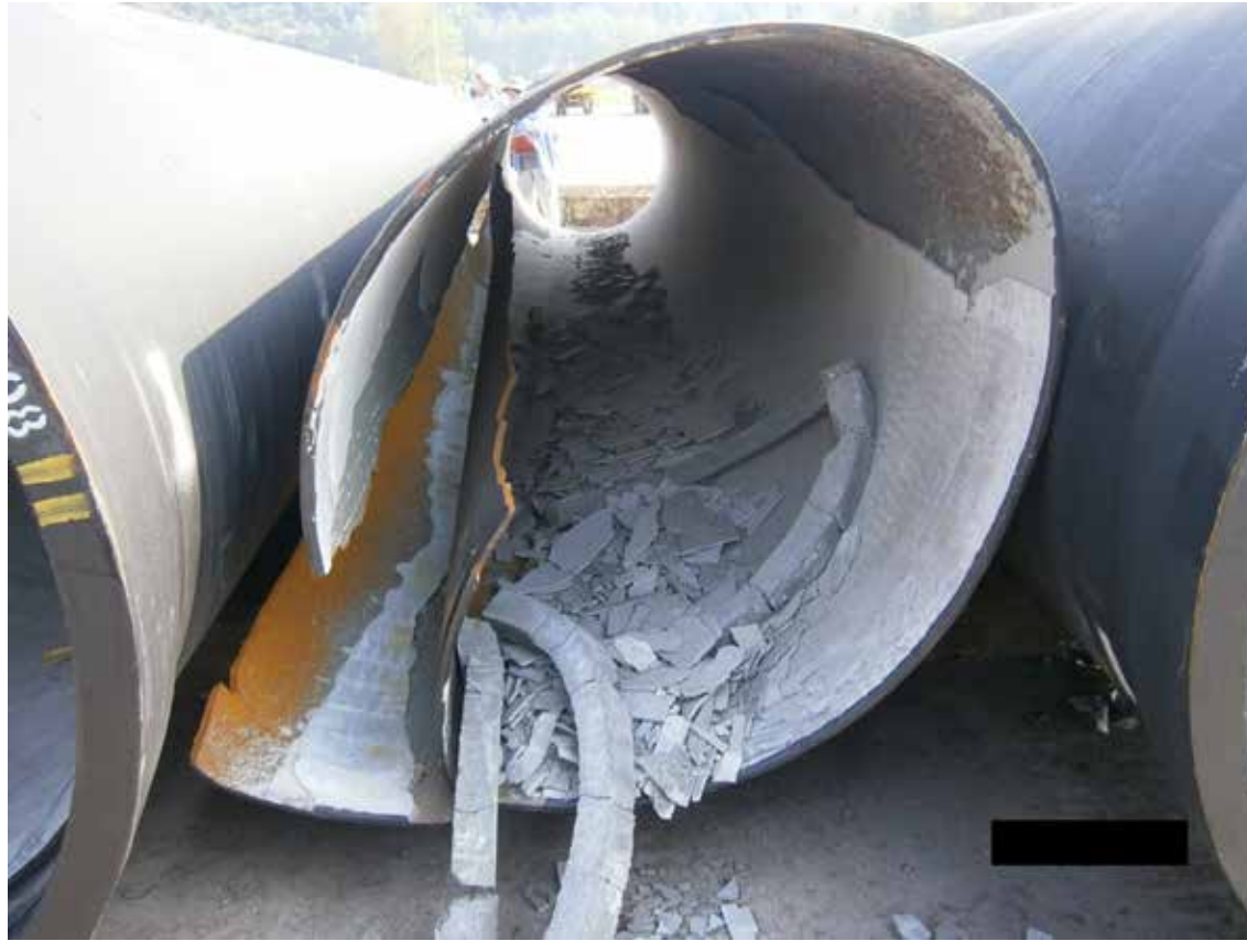
Compressed cast iron pipe
