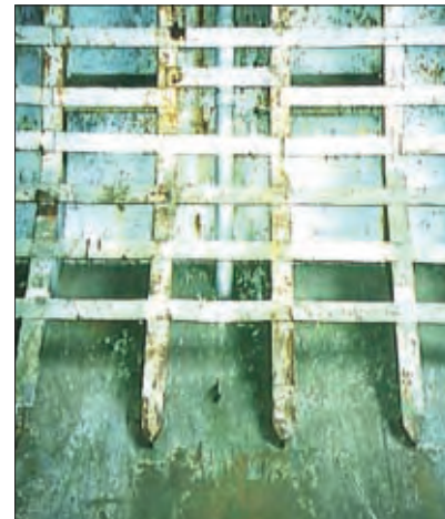
Figure 1: Spar ceiling in the form of strips of steel sheet fitted to the side frames.
