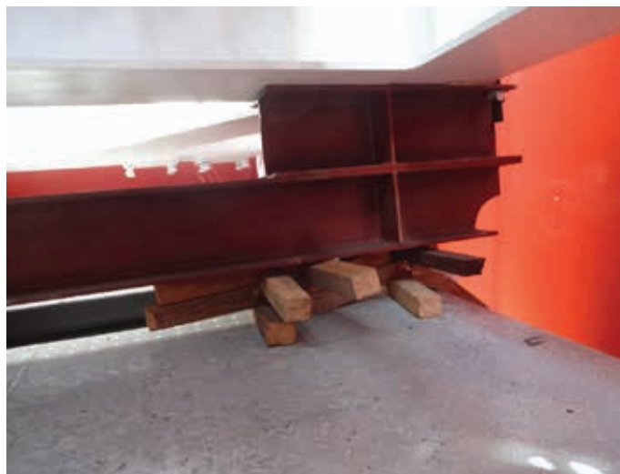
Figure 4.8 | Crushed dunnage due to improper arrangement.
