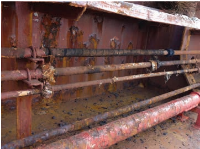
Figure 2.5 | Hatch coaming and deck piping in poor condition.
