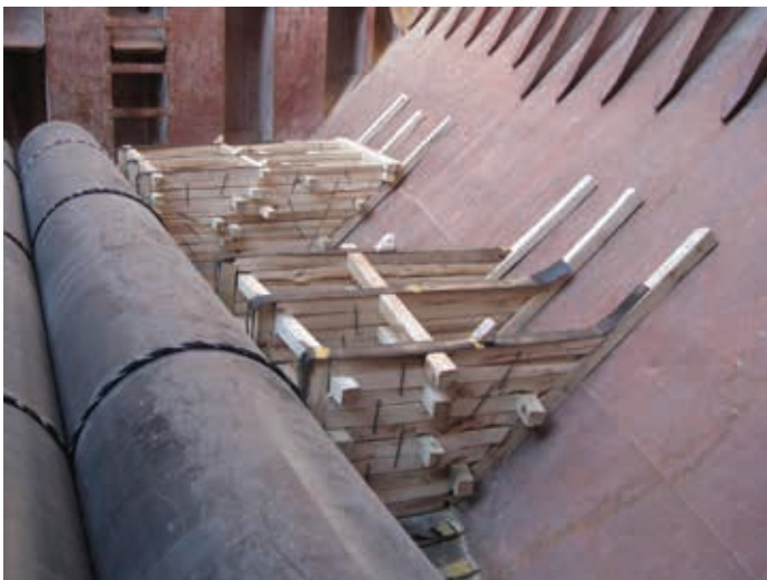
Figure 4.5 | Dunnage structures constructed on sloping hopper tank to hold large steel diameter pipes in place.
