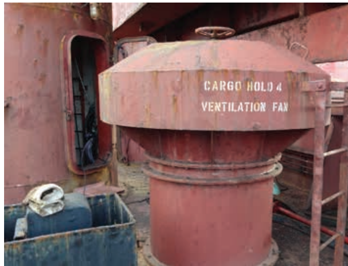
Figure 2.6 | Cargo hold mechanical ventilator.
