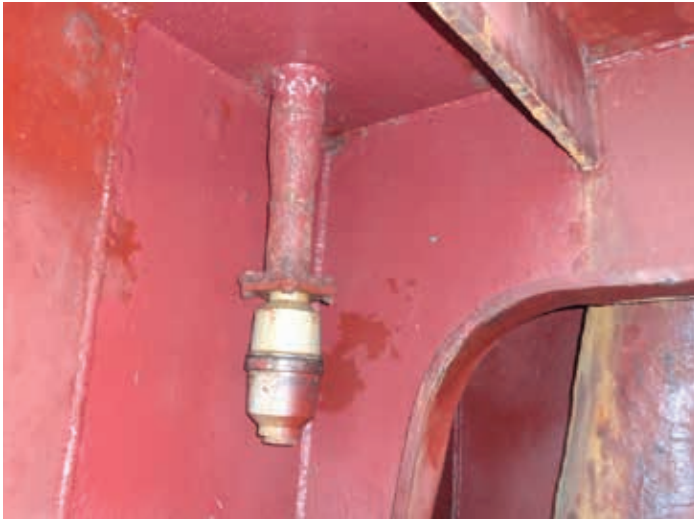
Figure 2.3 | Fire cap for the water draining non-return pipe is missing.
