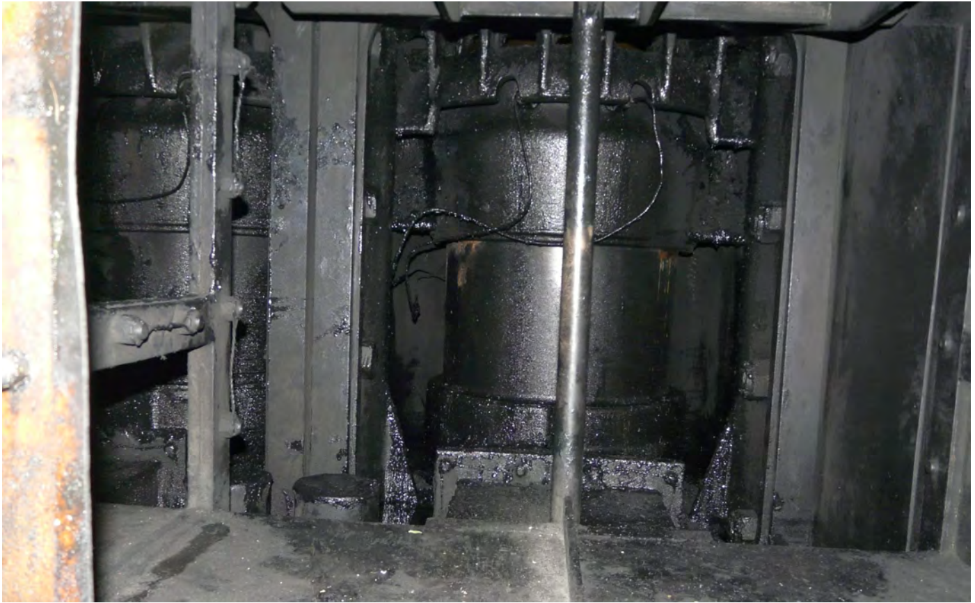
Figure 2.4 | Scavenge space charred after fire
