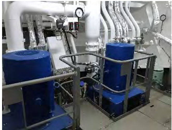
Figure 3.5 | Seawater pumps for scrubber system in engine room
