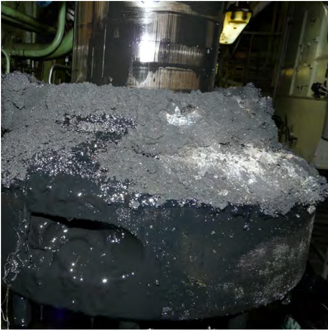
Figure 2.5 | Main engine stuffing box carbonized
