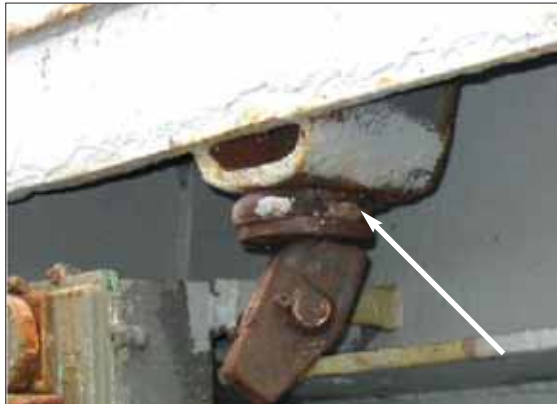
Overtightened rubber washer of quick acting cleat
