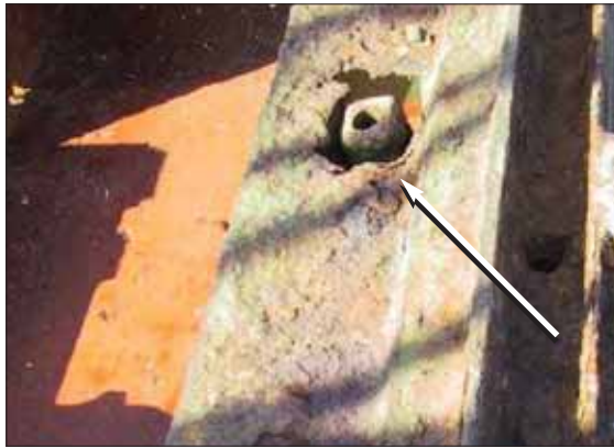
Coaming table in way of quick acting cleat cut-out reduced in thickness through corrosive action
