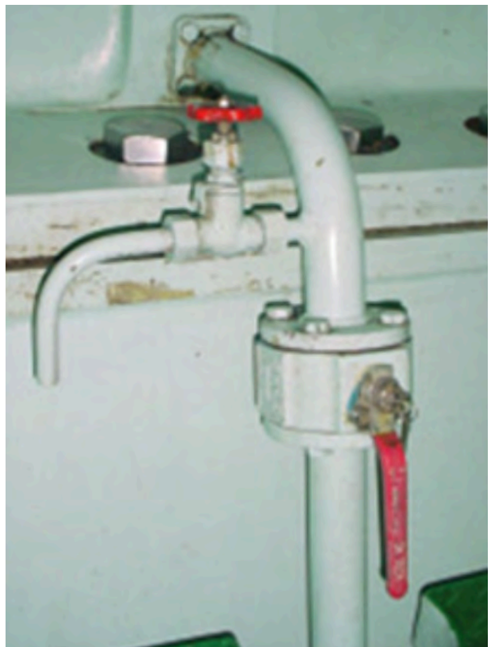
Photos 1 & 2: Sampling valves on the drain pipe - source CM Technologies GmbH
