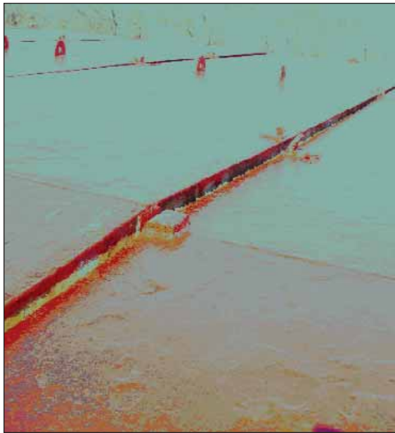
Misaligned hatch cover panels.
