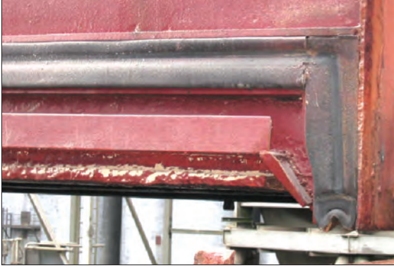
Excessive permanent imprint on packing rubber
