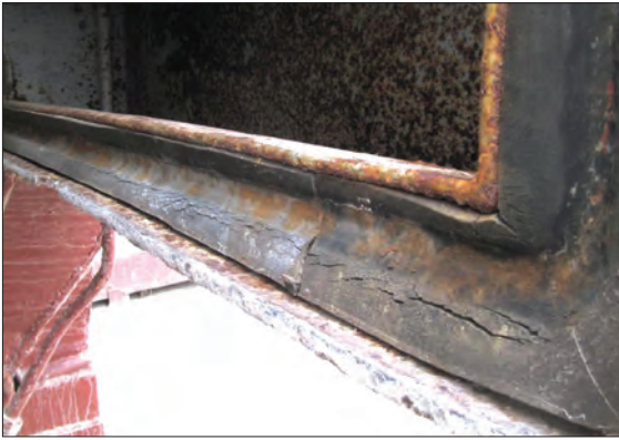
Overcompressed packing rubber with cracks becoming apparent in the sealing surface of the rubber
