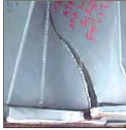
Cracked panel girder (stress crack)
