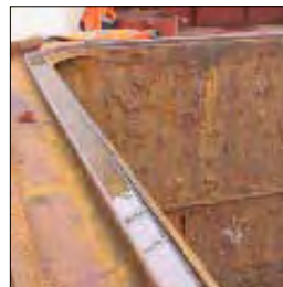
Blocked drain hole/valve, preventing water to be drained away to the deck
