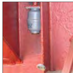
Original non-return type drain valve with fire cap secured with a lanyard
