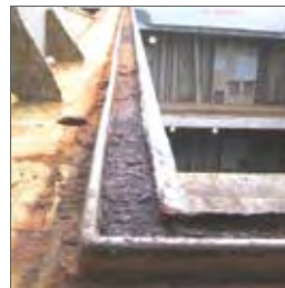
Accumulation of rust scale in drain channel
