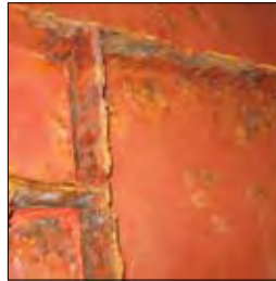
Corroded panel structure
