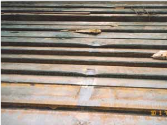
Figure 4: Indentations to flanges caused by hard timber dunnage.
