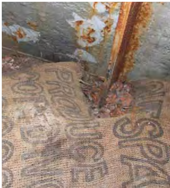
Figure 4: Mould damage where a bag in (3) has come into contact with the shell plating.
