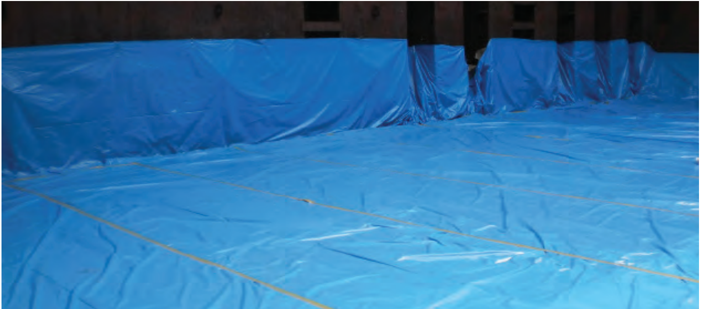
Figure 3.9 | Kraft paper overlaid with plastic sheeting on the tank top and continue vertically along the corrugated transverse bulkhead.
