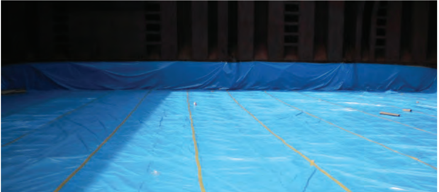
Figure 3.6 | Kraft paper overlaid with plastic sheeting on the tank top. This continued vertically along the corrugated transverse bulkhead in background.
