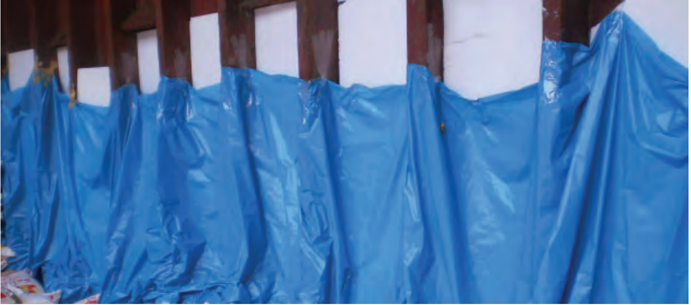
Figure 3.7 | Styrofoam laid between sideshell frames and then overlaid with blue plastic sheeting.
