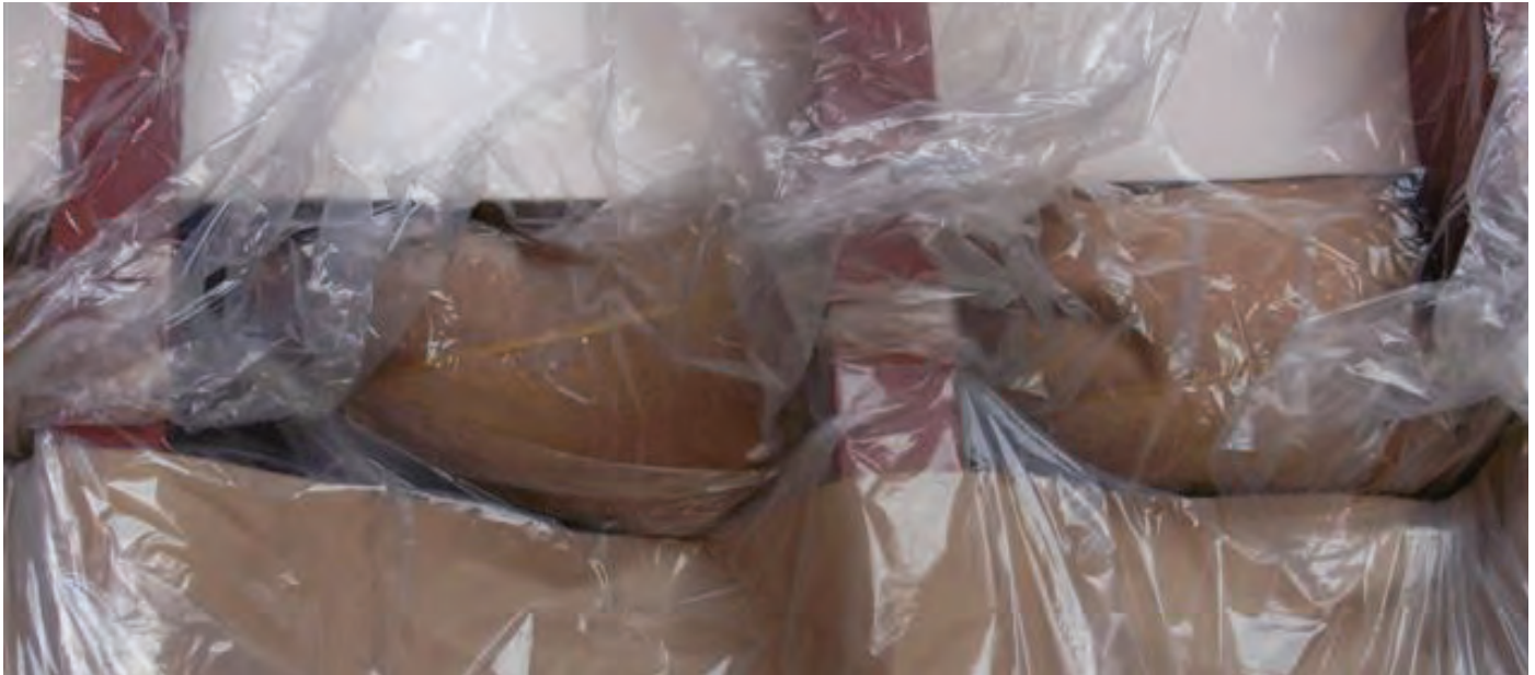
Figure 3.17 | Saw dust in burlap bags is inserted at transition point between sideshell and top of hopper tank. Notice the Styrofoam sheets above and kraft paper beneath the bags is then overlaid with plastic sheeting.
