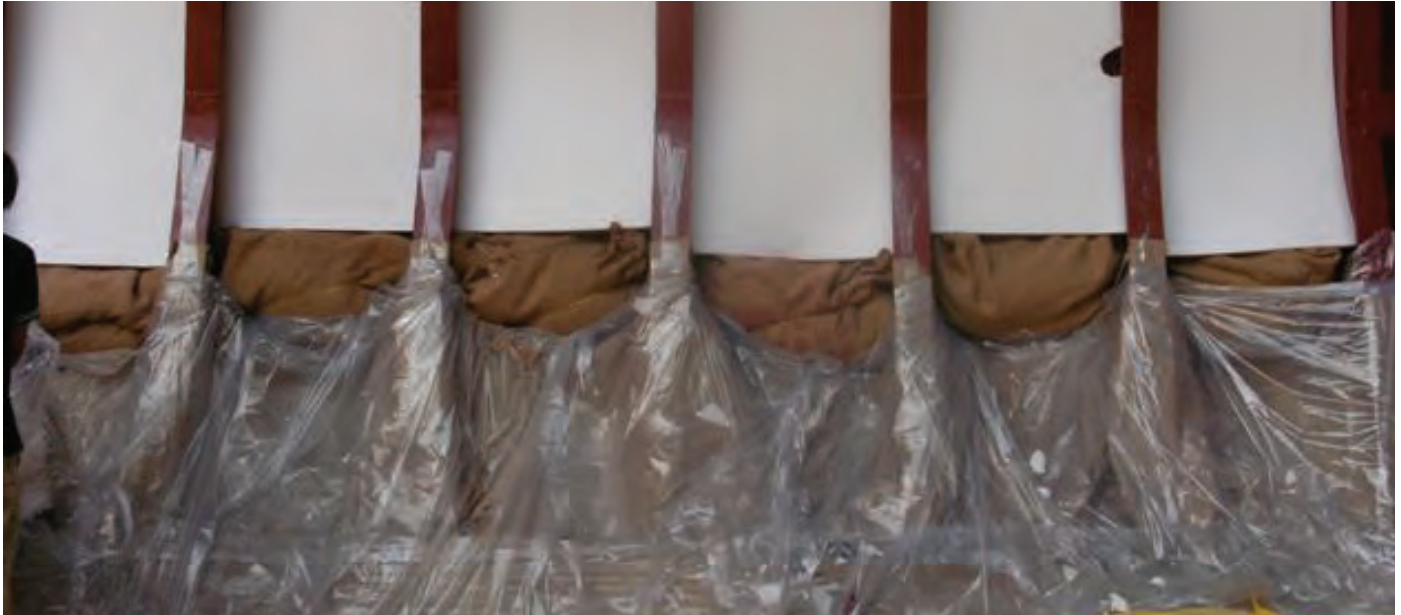
Figure 3.18 | Saw dust in burlap bags is inserted at transition point between sideshell and the top of the hopper tank.
