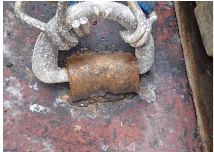
Cargo securing point in poor condition.
