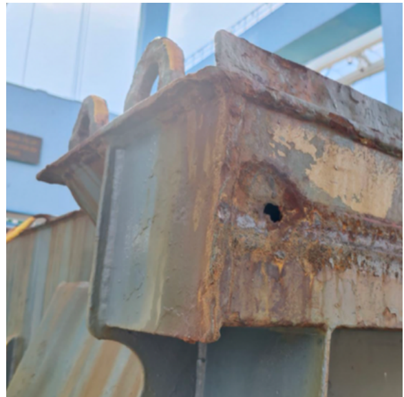
Hole in a hatch cover through which water entered the cargo hold during heavy weather.
