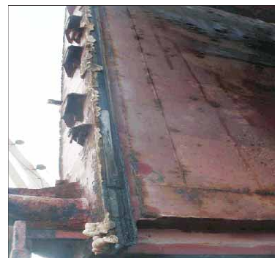
Worn packing additionally sealed with mastic and foam.
