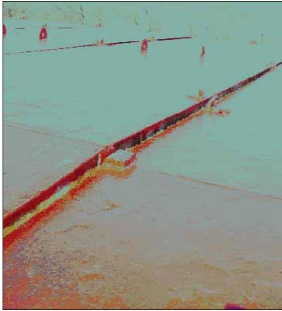
Misaligned hatch cover panels.
