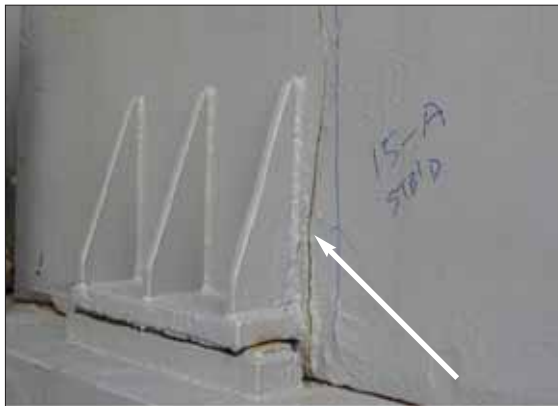
If bearing pads can not move/slide over their mating surface, cracks will occur in the side plating or...
