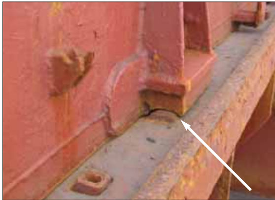
Worn bearing pad, causing over-compression of packing rubbers and undue stresses on panel hinges, wheels,...
